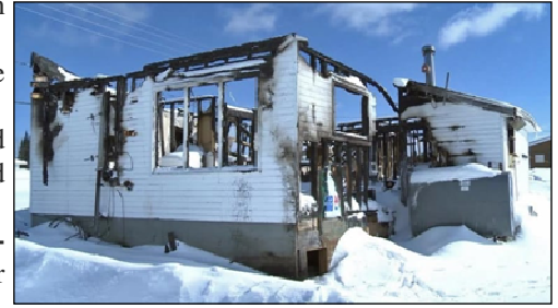
The chief of Mishkeegogamang First Nation sought a coroner's inquest to expose inadequate funding for fire protection and housing after a fire in this house killed four people in February 2014.
